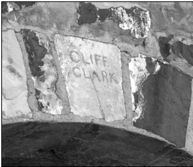
Figure 13: Clifford Clark was the foreman of the Cat Creek bridge project in southwestern Prowers County. Photo: Deon Wolfenbarger, June 2004.
