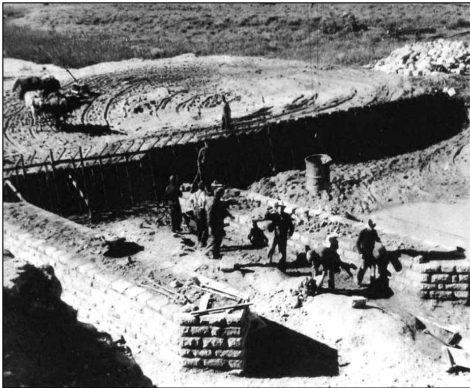
Figure 10: Example of the intensive hand labor that went into the construction of the Bear Creek Bridge in Baca County; 5BA.788.
