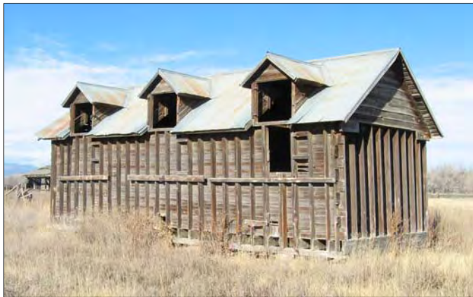
The Keyes granary at 9748 N. 119 th Street—a rare studs-out granary with dormers. The dormers are used for filling the structure with grain.
