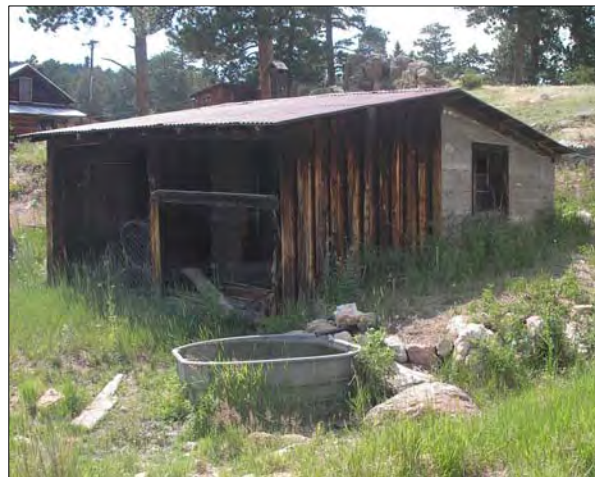
Concrete block springhouse with wood addition built into the hillside at Scates Ranch on Magnolia Road, with a pipe leading to a stock tank.
