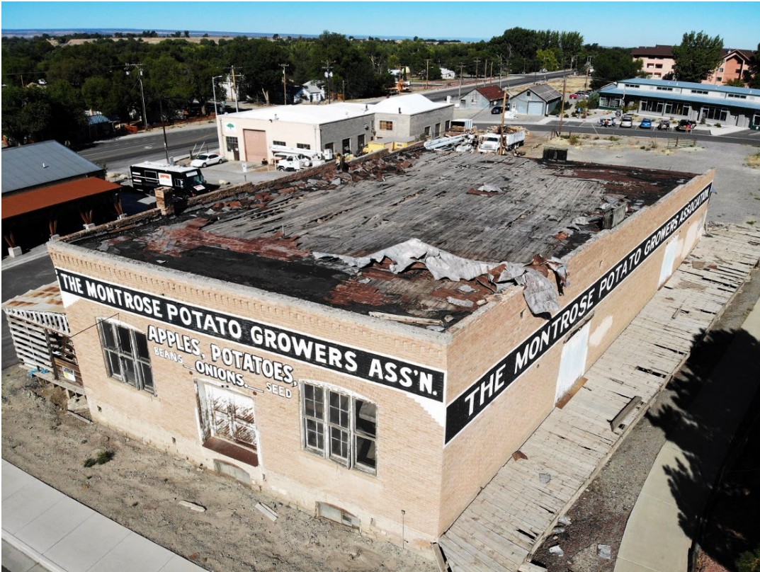
Figure 8: Aerial photo taken (25 September 2019) prior to 2019 rehabilitation, camera facing northwest. (Source: William Woody)
