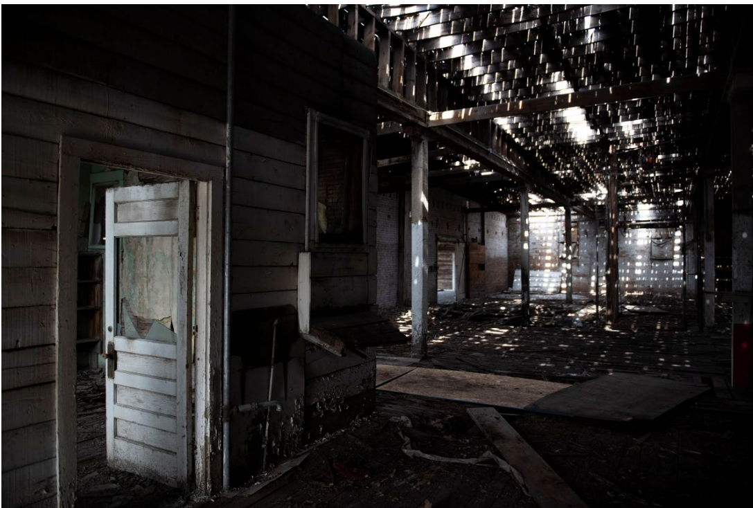
Figure 9: Photo of interior taken (10 October 2019) prior to 2019 rehabilitation. Office to the left (no longer extant). (Source: David Fishing)
