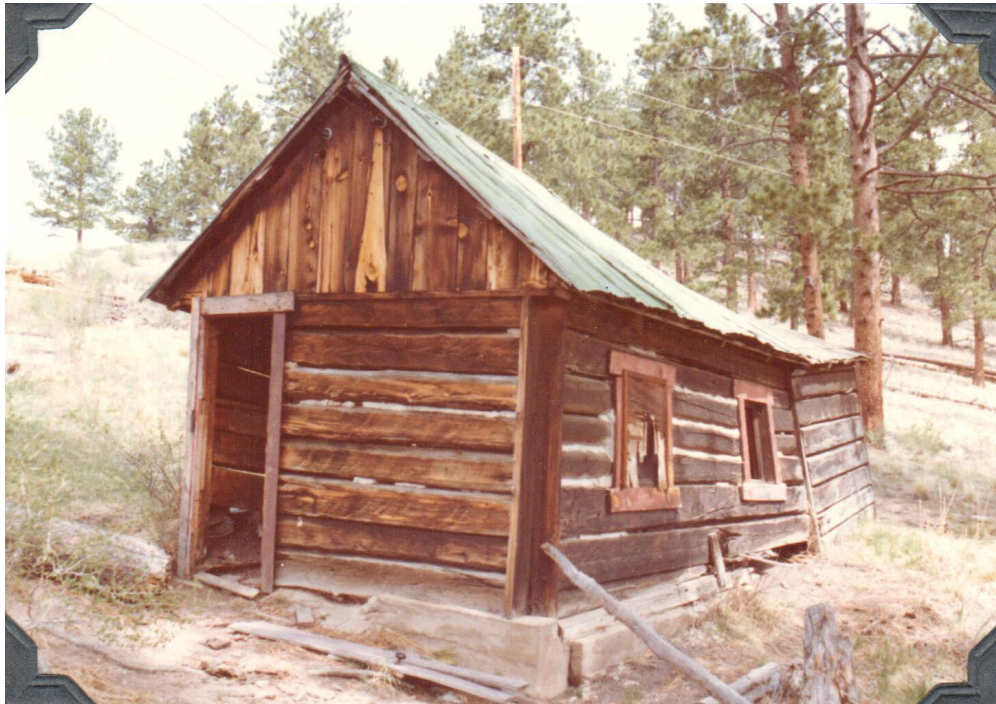
Photo HP3. Generator House, view to the northwest, showing the south and east façades, (Dargan 1979).
