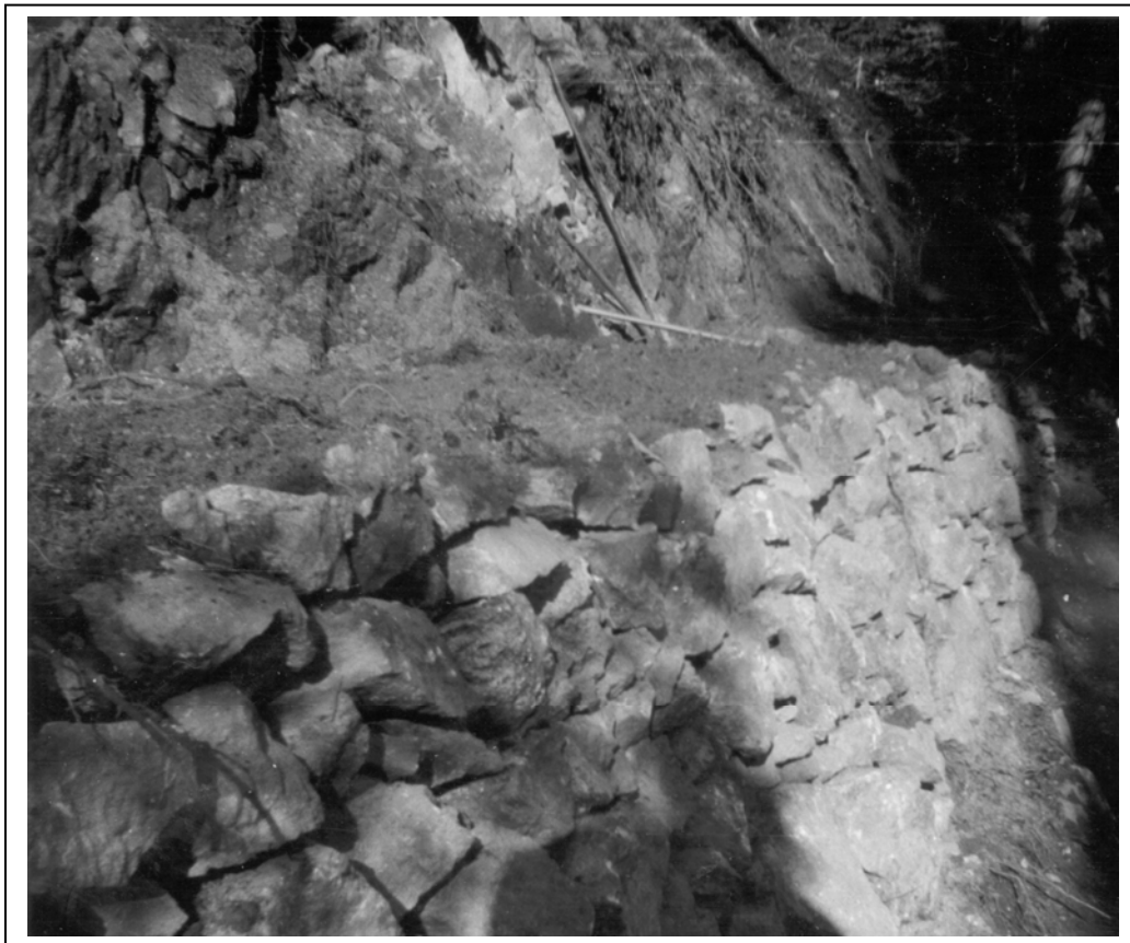
Stone Wall along North Inlet Trail Courtesy of Rocky Mountain National Park Taken by Edward Ramalay, 1929-1930
