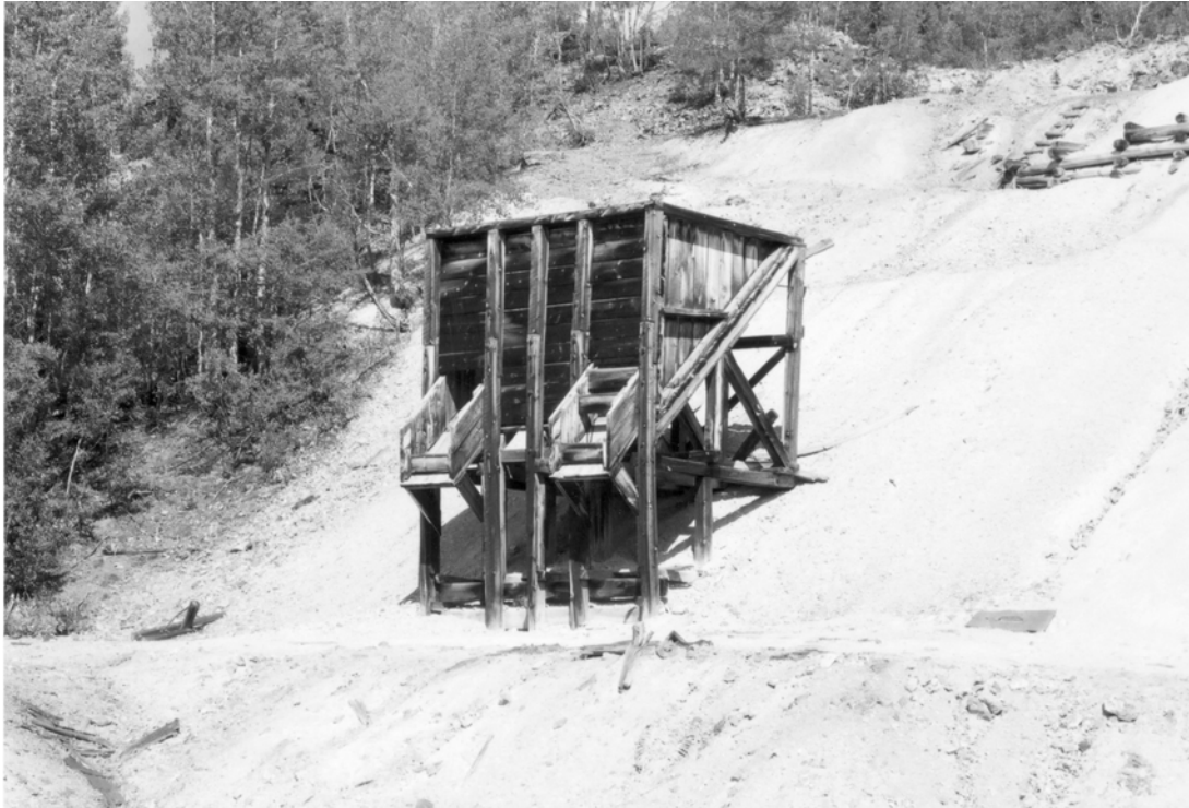
Fig. E.II.53 A typical sloped-floor ore bin. Miners emptied ore cars into the open top and workers extracted the ore through the chutes when hauling it away. Eric Twitty, Red Mountain Mining District, taken 1998.
