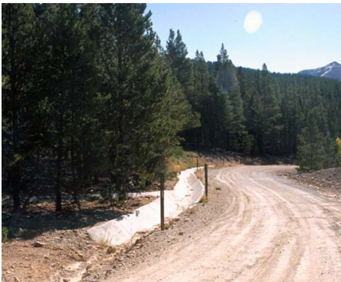
Fig. E.I.22 Concrete culvert used in environmental Remediation in 2005. Collection of James E. Fell.
