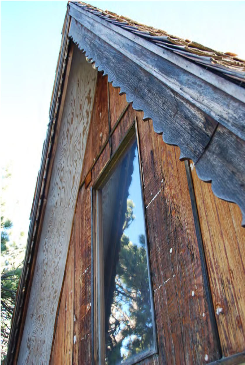
128 Cabin Creek Photo by J. Wahlers 11/2/2017 Detail of scalloped bargeboard and upper gable window
