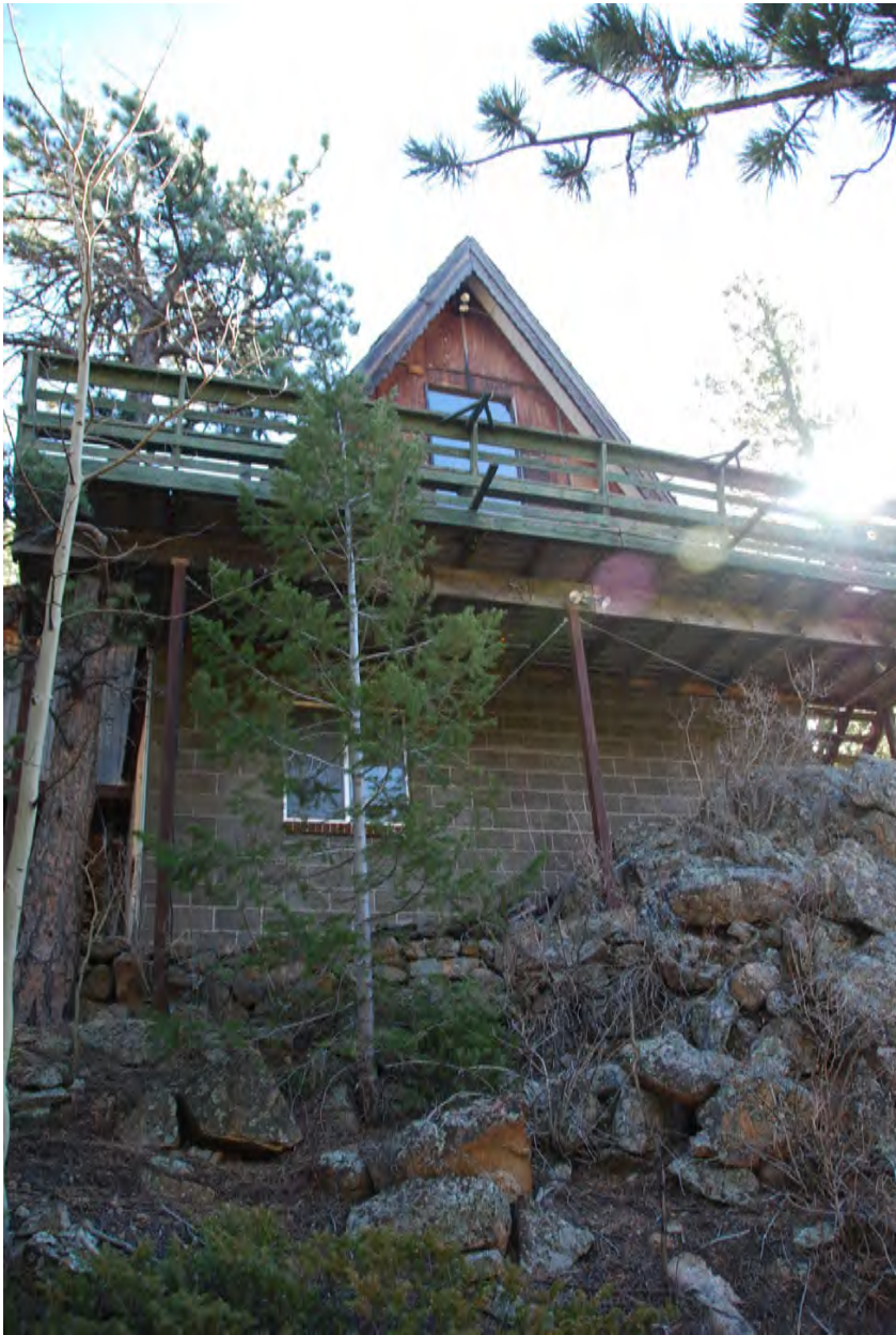
128 Cabin Creek Photo by J. Wahlers 11/2/2017 View of front elevation from below
