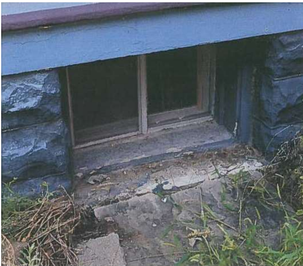
Figure 7: Basement window prior to alteration to create new egress. Photo from September 7, 2016, Design Assistance Program application filed by Alan Braslau and Nathalie Rachline with the City of Fort Collins. (Fort Collins Historic Preservation Division).
