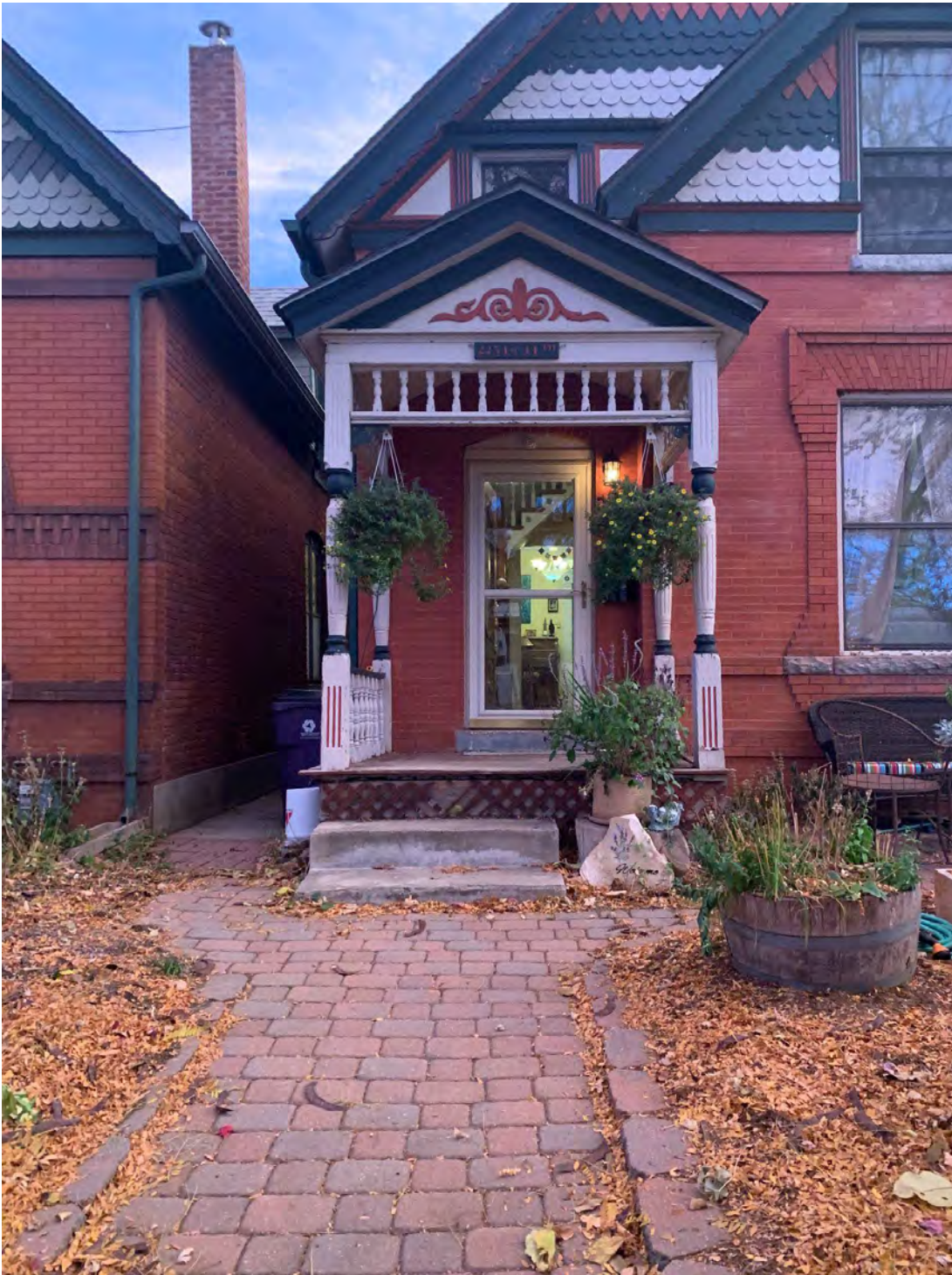
2. View of covered porch entry with turned spindles, carved-wood address placard, and ornamental fascia design. Photo taken November 5, 2022.
