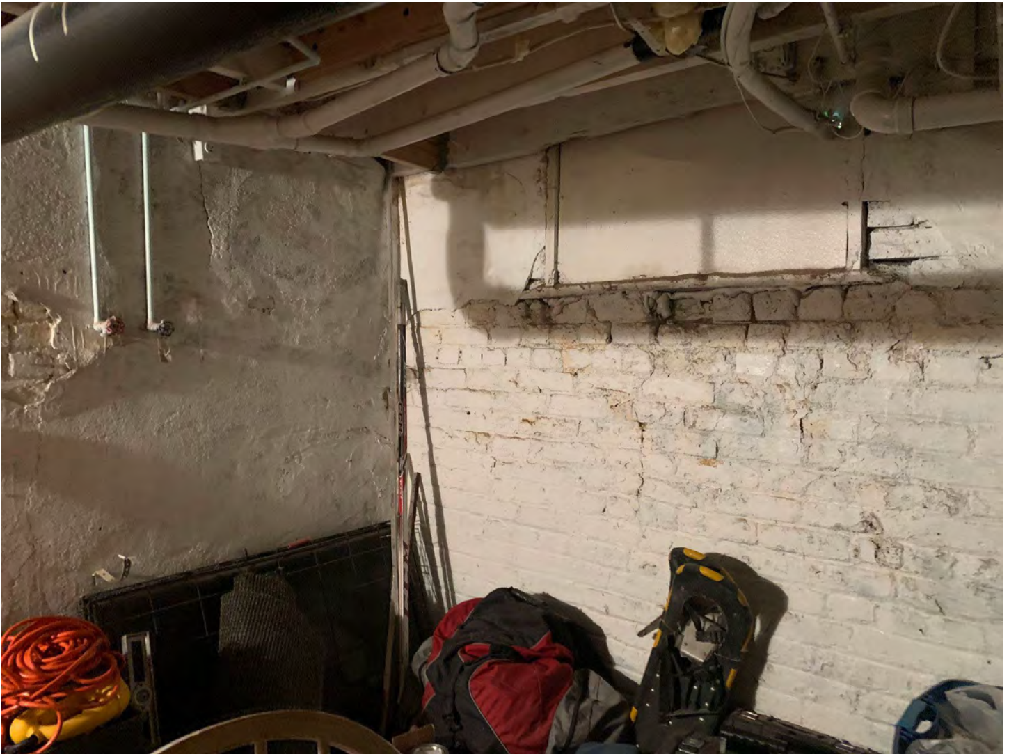
37. Cellar brick wall with some plaster repair. The boarded window faces south into the backyard. The white finish is mold remediation paint. Photo taken September 26, 2022.
