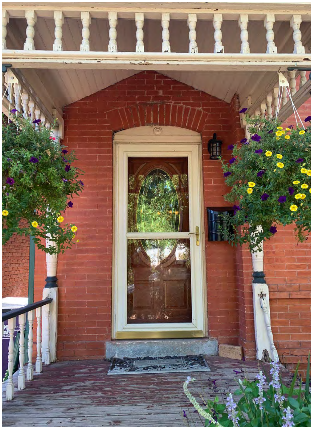
3. View of the front porch entry and door. Note the brick semi-arch above the door frame. Photo taken September 26, 2022.
