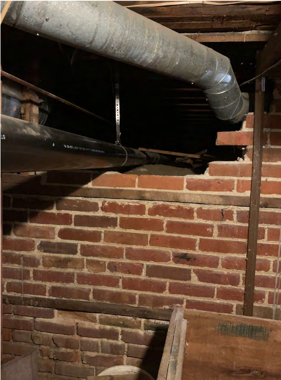
36. Cellar crawl space entry. Photo taken September 26, 2022.
