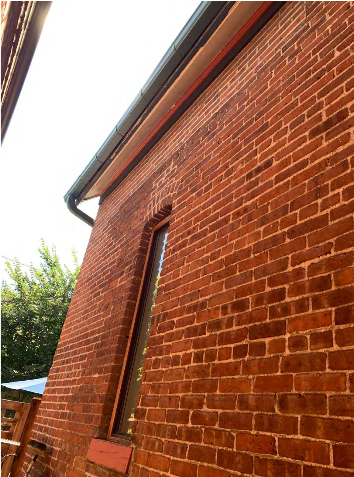
7. Photo noting layer of new brick delineating the second floor main bedroom addition. Includes first floor bathroom east-facing privacy window with new wood frame (ca. 2017). Photo taken September 26, 2022.
