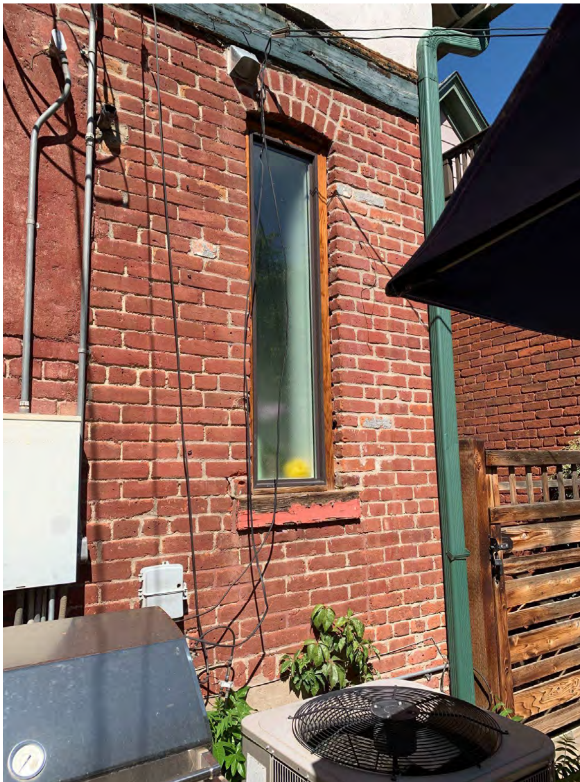
12. South-facing first floor bathroom privacy window with new wood frame (ca. 2017). Photo taken September 19, 2022.
