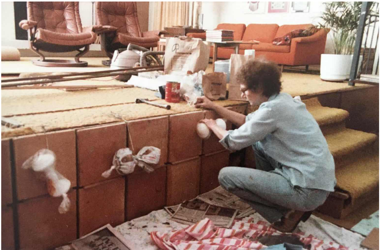
10 of 16: Patterson Home, Jo Patterson tiling living room platform, 9841 Rapp Lane, date unknown.
