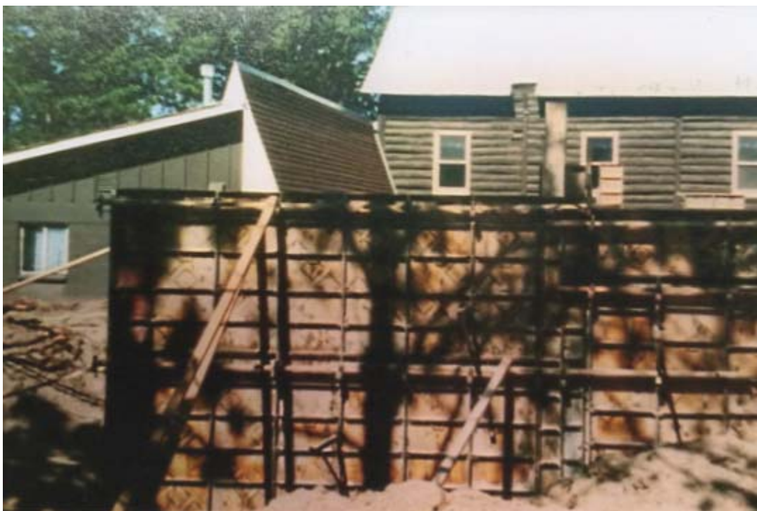
Historic Photo 2- Log Building, East Side, showing 1953 Basement Addition (behind Morast Hall construction)
