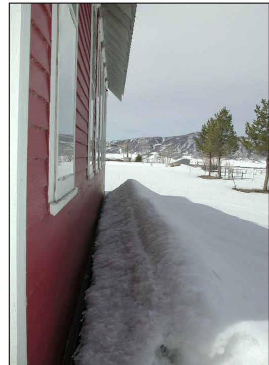
Sources of moisture, such as snow piles, should not be allowed to collect against foundation walls.
