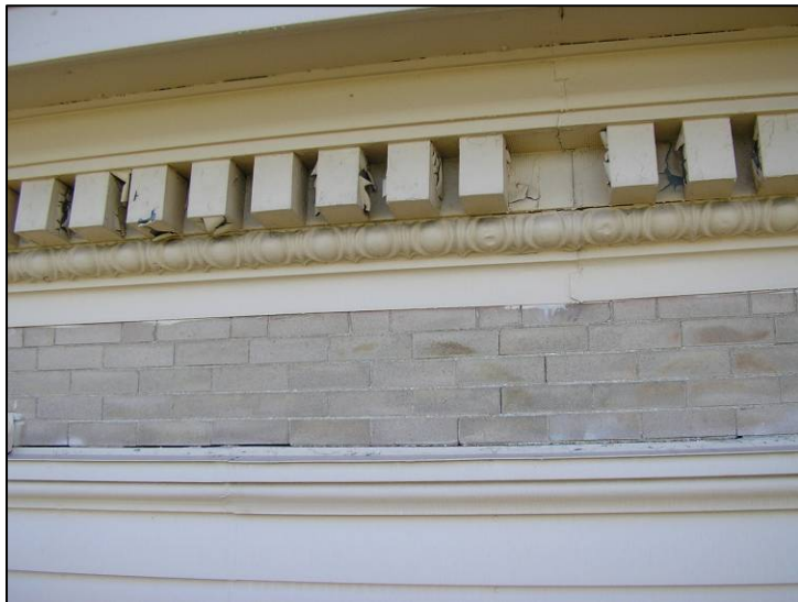
Building features such as these cornice dentils are important to maintain in order to avoid losing character-defining elements.
