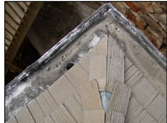
Missing or damaged shingles should be replaced as soon as possible.
