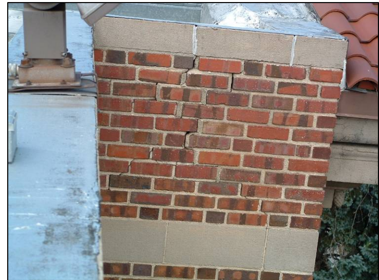
Masonry parapet walls are prone to moisture damage, such as deteriorated mortar joints, and should be examined regularly.
