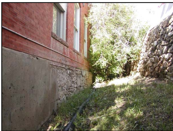
Ground that slopes towards the building foundation will bring unwanted moisture and should be addressed.
