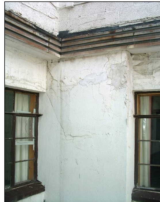
Cracks in stucco should be repaired to avoid moisture entering and enlarging them.
