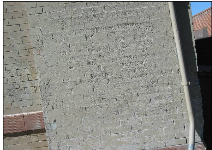
Destructive cleaning techniques such as sandblasting can damage masonry and other materials and should not be used.
