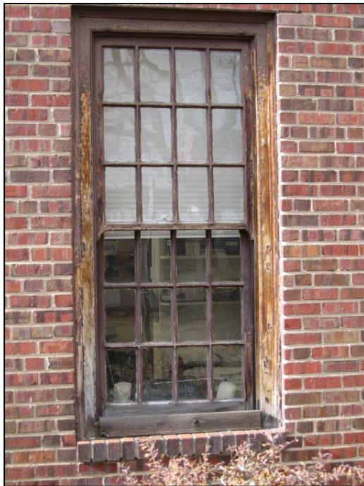
Lack of maintenance painting has caused this window to weather severely.
