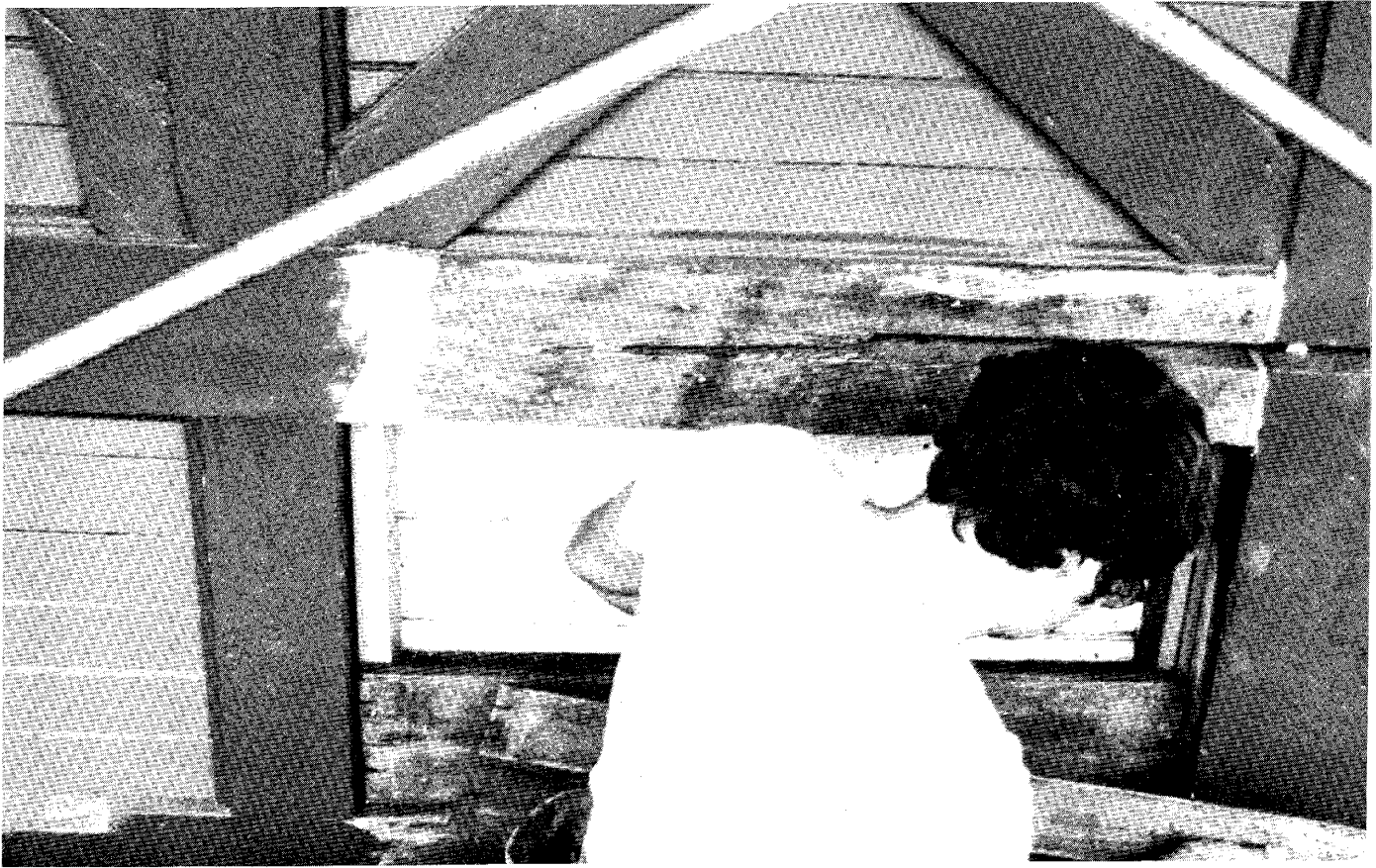
Figure 6. Sound pieces of wood salvaged from elsewhere on the building are being used to replace this deteriorated tongue and groove panel. In most cases, deteriorated wood trim, sills, and paneling were replaced with redwood that was back primed. Photo: Bryan Blundell
