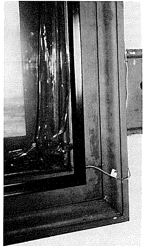
Figure 2. The thin-framed storm unit is shown attached by a magnetic seal to the existing trim. The protective film on the acrylic will later be removed. Photo: Tom H. Taylor.
