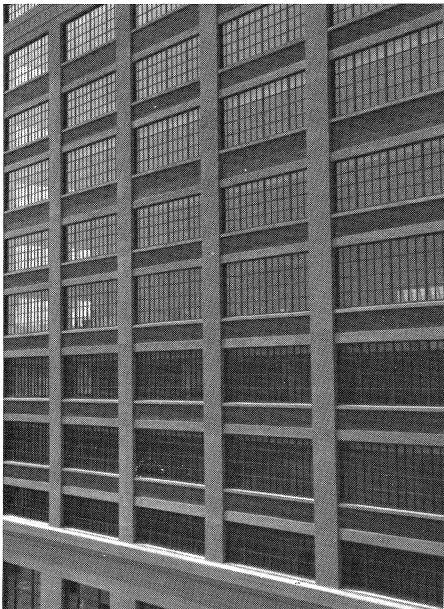
Figure 8. The window work at 149 Constitution Park represented a significant improvement over past attempts to recapture the distinctive qualities of a steel industrial window with narrow-bead glazing bars, using an aluminum replacement system with insulating glass. Success was achieved through careful and well coordinated planning. Photo: Charles Fisher.
