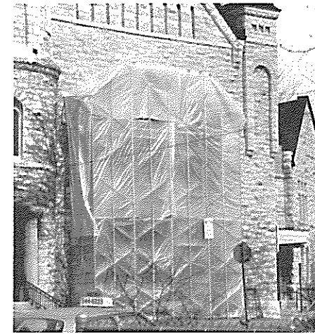
Figure 3. A vinyl cocoon placed over the windows allowed the repair work to be carried out even in inclement weather.
