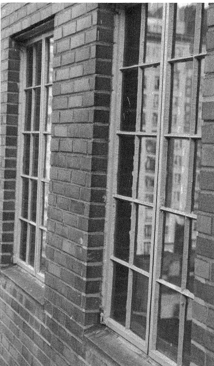
Figure 7. The dark frame color and careful installation of the interior storm window resulted in little visual impact on the exterior appearance of the building. Photo: Charles Fisher.
