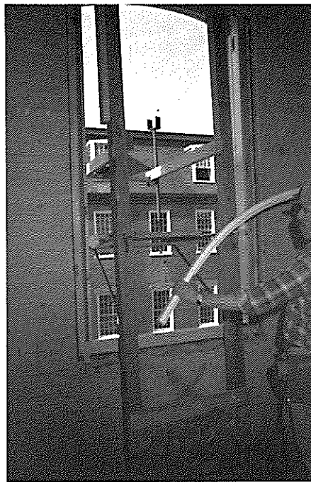
Figure 7. "Gun carriage" (scaffolding) in use by the window re-installation crew who are preparing to replace missing brickmold with replacement made by the millwork shop. Note saw kerfs used to create arc in molding for use in the window head (same method as used in the original molding). Photo: Christopher Closs
