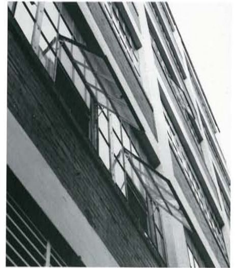
Figure 7. Retrofitted projecting ventilator with the TRUTH hinges. Photo: Robert Powers.
