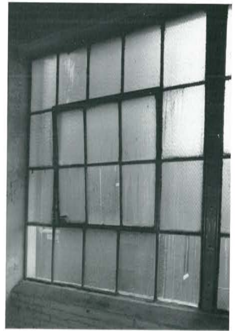
Figure 1. Typical multi-light steel window with ventilator as seen from the interior. This window exhibits typical pre-rehab conditions including silt corrosion, missing hardware and a poorly operating ventilator. Photo: Clio Group.
