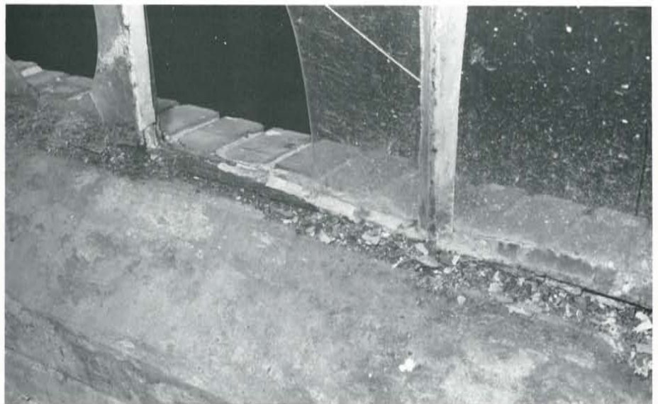
Figure 5. Sill corrosion typically found on 95% of the windows. Photo: Clio Group.
