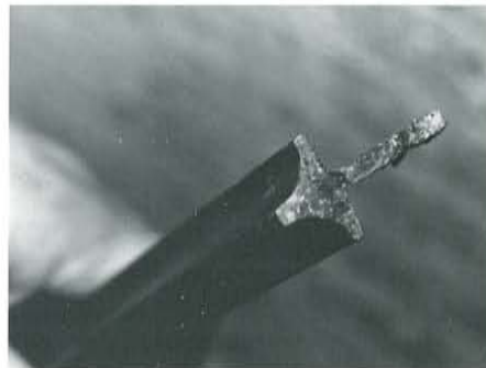
Figure 10. Replacement steel window section used primarily in the sill areas. Photo: Clio Group.
