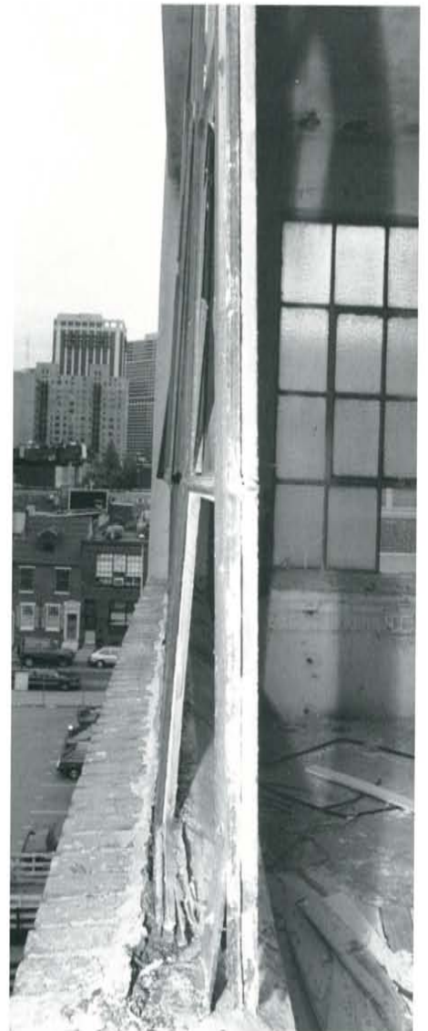
Figure 8. Bowed and corroded window during construction. Photo: Clio Group.
