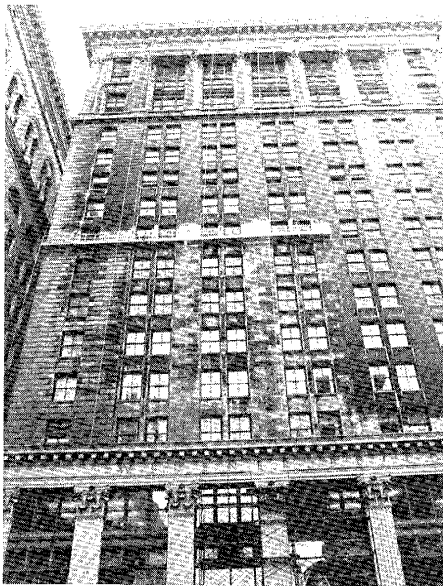
Figure 4. South Penn Square elevation after the completion of two drops from the 9th-4th floors of water soaking only, and prior to beginning the rinse process. Photo: P & R Masonry Restoration, Inc.
