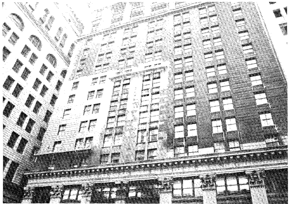
Figure 5. The drop on the left side of the building has been water-soaked and rinsed, while the drop on the right has been soaked only. Note the amount of soil that still remains on the right side before rinsing. Photo: P & R Masonry Restoration, Inc.
