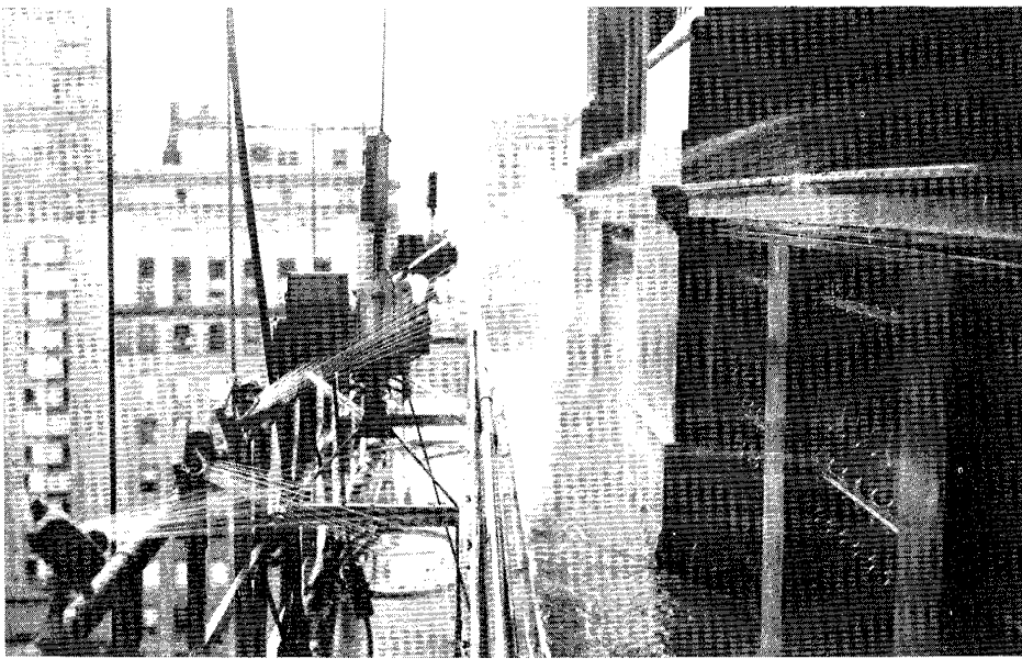
Figure 3. Close-up view of the oscillating sprinklers spaced 3 feet apart and connected to 1/4" PVC piping attached to the rear bar of each scaffold. Photo: P & R Masonry Restoration, Inc.
