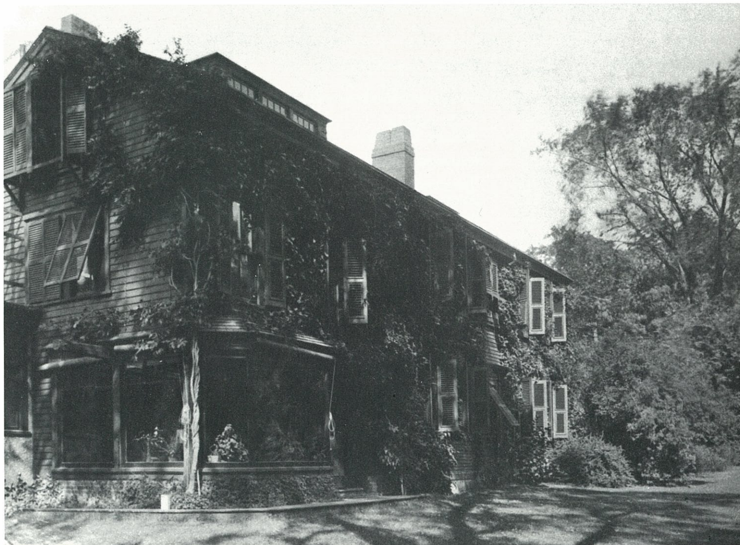
Figure 2. View of the west elevation at Fairsted which shows a steel strapping trellis system built as early as 1884. Photo courtesy of Olmsted National Historic Site.
