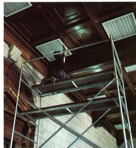
3. The light fixtures were carefully removed to permit installation of a sprinkler system behind the coffered ceiling and to restore the ceiling to its original appearance. It was necessary to reproduce 40 new panels for installation in the coffered ceiling, due to the damage resulting from the 1962 lighting work. Photo: Dell Corporation
