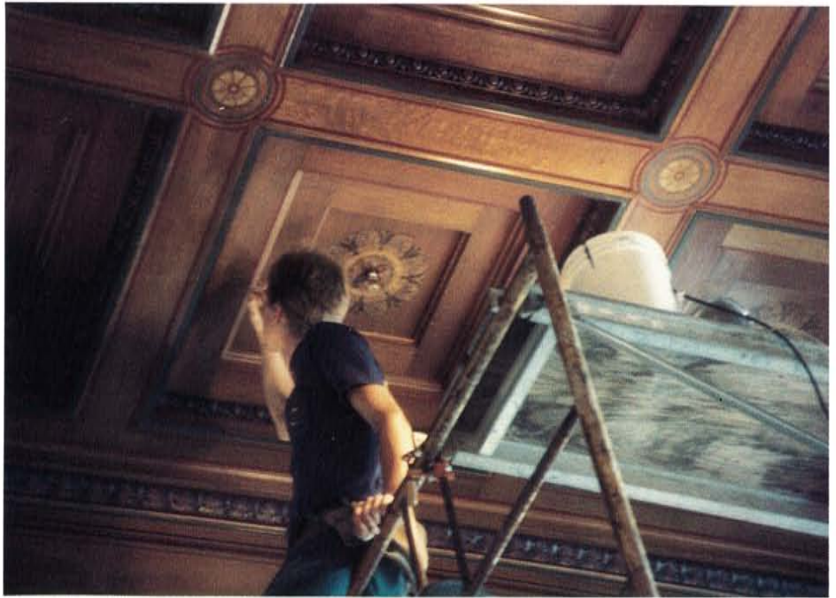
6. The finished panels were installed in the ceiling with new sprinkler heads located in the center of the cherry motif. Stainless steel pins were used to set the panels, since there was no room to lift the panels in place from above the ceiling once the wet piping system was in place. Photo: Dell Corporation.
