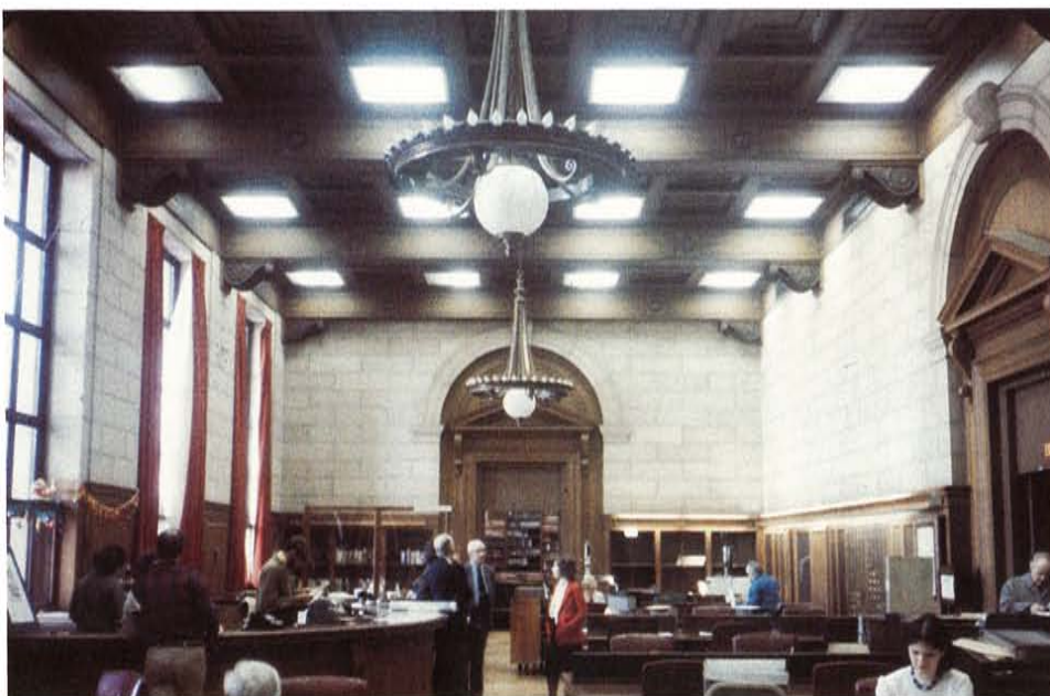
2. The 40 large visually obtrusive fluorescent lights, installed in 1962, damaged the coffered ceiling in the Central Search Room. Photo: Dell Corporation.
