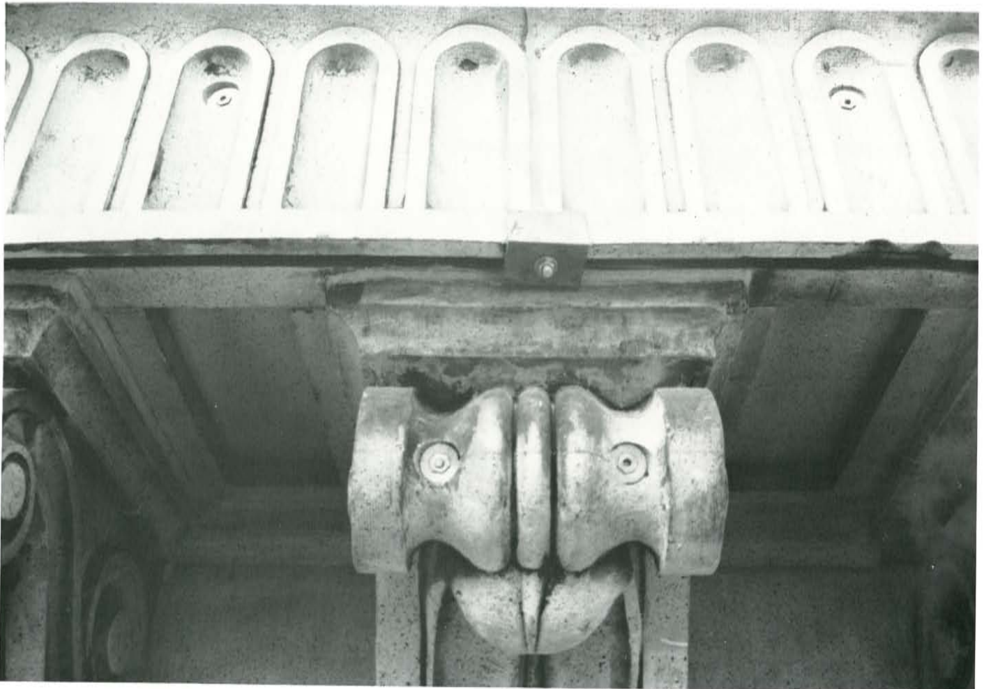
Figure 11. Completed anchor installations at a fascia and bracket. The countersink holes penetrate no more than half the thickness of the outer wall of the terra cotta and were filled later with epoxy.
