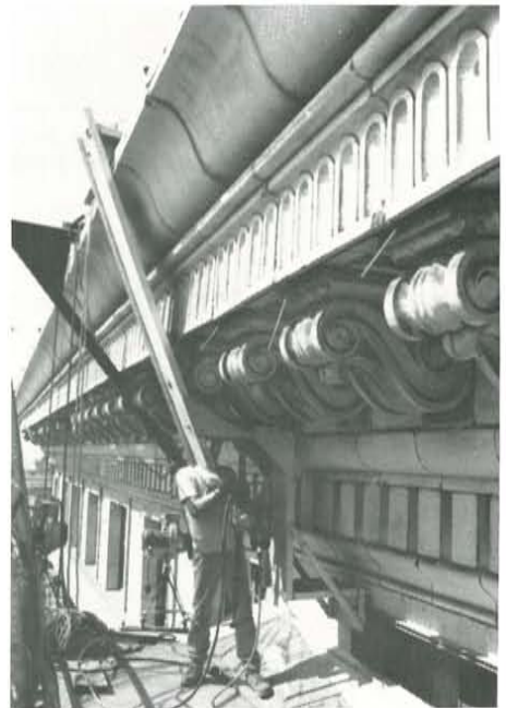
Figure 9. Drilling 6' long vertical holes through the cornice, in a variety of materials, was a delicate operation requiring great skill and specialized drilling equipment. The aluminum drilling jig provided the precise alignment needed to drill the holes for the vertical and angled bracket anchors. Drilling of a vertical anchor is shown. To create an angled outer scroll anchor hole, the drill was mounted on the angled portion of the jig, which passed directly in front of the bracket. Hand-drilled holes could be completed in 15-30 minutes, depending on the depth of the hole and the type of backup material encountered (e.g., brick, terra cotta, light-weight concrete, steel). Holes drilled with the jig required more time, 30-60 minutes, as alignment was more critical and it took time to set the jig in the proper position. Photo by Jeffrey S. Levine.
