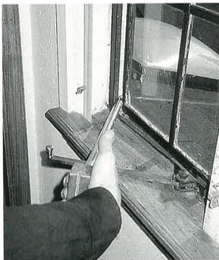
Figure 6. Pull bars were used to realign the sash from the inside. These custom made tools were especially useful on single sash units where the worker was unable to reach through an adjacent opening to apply pressure from the outside.
