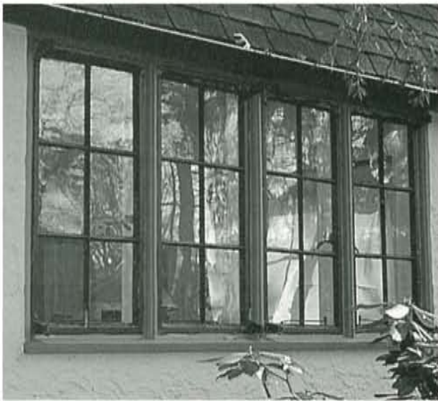
Figure 2. Each casement sash had six lights with projecting hinges that allowed the unit to open outward. Note the variation among glass panes as seen in the reflections. Caused by small differences in the positioning of panes within the sash and minor imperfections in the glass itself, this appearance is an important characteristic of historic windows.
