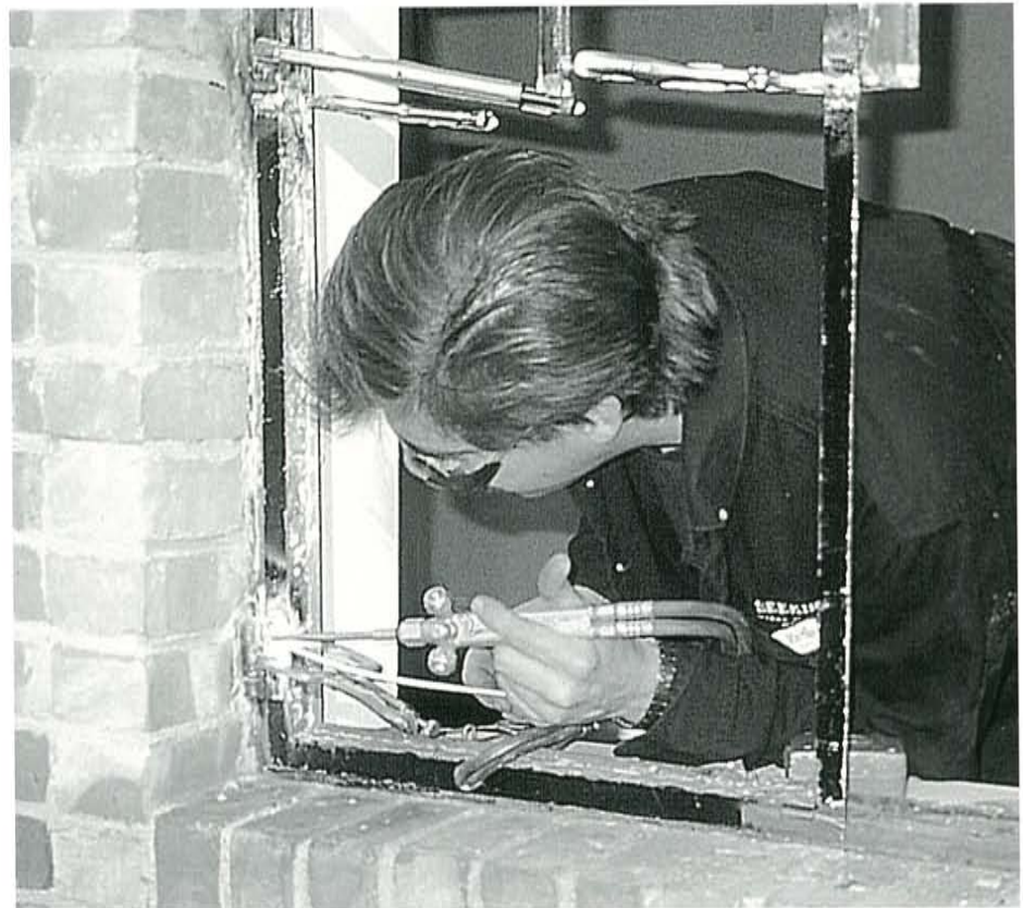
Figure 7. New steel sections were brazed into the historic sash and frame where the windows had previously been altered to fit air conditioning units. Because the replacement pieces came from a stock of salvaged window materials, they matched perfectly the profiles and dimensions of the missing sections.
