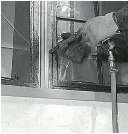
Figure 8. A pneumatic needle gun was used to strip much of the paint from the steel frame and sash. It was followed by wire wheel and small disk sanders and hand chisels. The blunt tipped needles did not damage the steel or adjacent glass.
