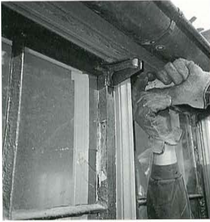
Figure 5. Before realigning the window, paint, caulk, weatherstripping and rust were stripped from all surfaces where the sash and frame were in contact.
