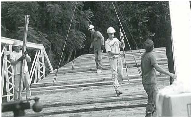
Figure 11. As the deck was lifted off the trailer and onto the floor beams, workers wedged timbers and bars along the sides to prevent the deck from damaging the truss and to help place the deck in position.
