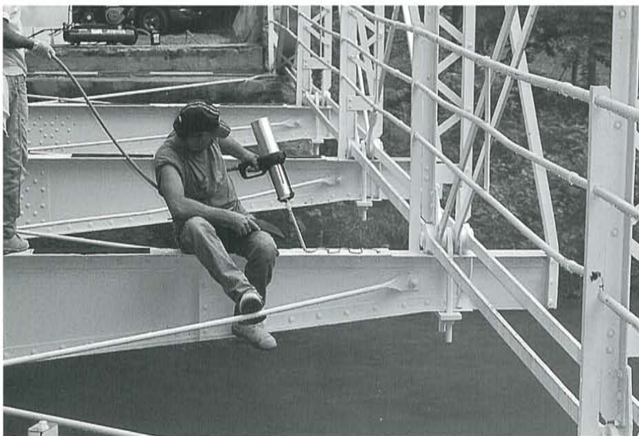
Figure 9. A worker applied adhesive to the floor beams where each of the bearing pads would be positioned. Four pads were installed on each floor beam to cushion the deck, evenly distribute loads to the floor beam and provide a secure fit between beam and deck.
