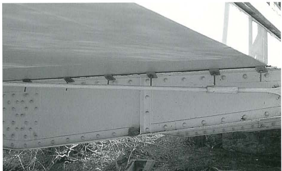
Figure 12. To secure the deck to each floor beam, lag bolts with steel clips were inserted into predrilled holes in the deck surface and fastened tight against the floor beam's upper flange.
