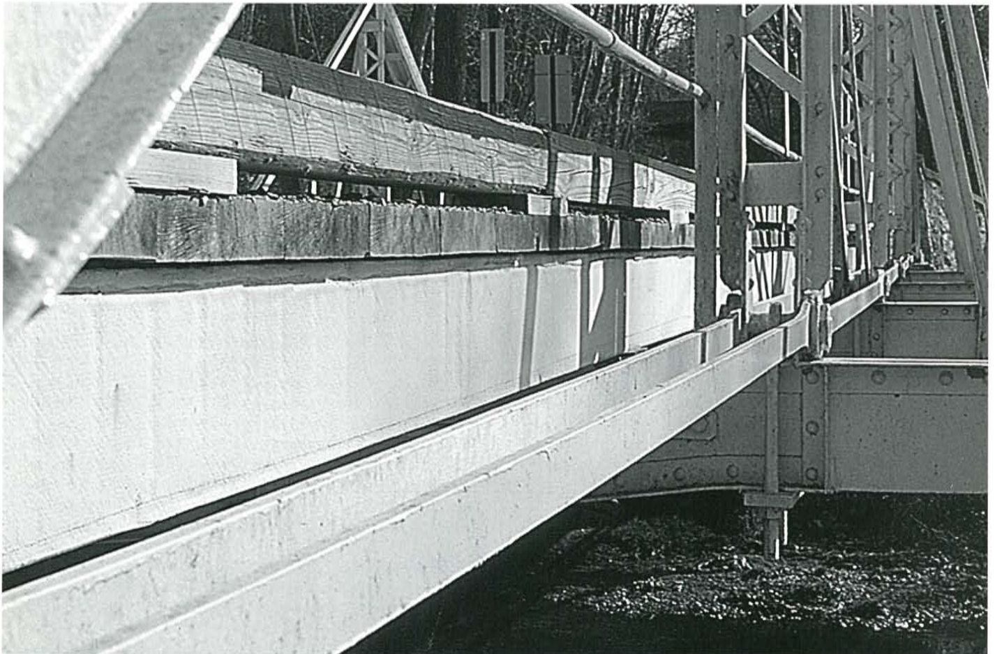
Figure 14. The composite deck, painted to match the superstructure, is visually compatible with the historic bridge as it originally appeared with timber stringers. The new deck and wearing surface are the same thickness as the previous system of steel stringers, nail-laminated deck, and bituminous surface. Photo: Chad Randl.
