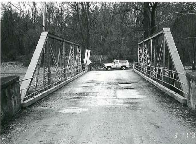
Figure 2. Before rehabilitation, Wilson's Bridge had an asphalt wearing surface that was delaminating from the deck below. Extensive cracks and numerous potholes were also present.
