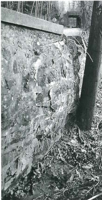
Figure 4. The Wilson Bridge wingwalls had loose and crumbling mortar joints. Much of the wall surface required removal of this deteriorated material and significant repointing.
