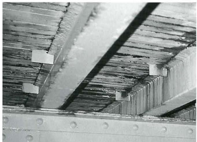
Figure 3. A view of the underside of Wilson's Bridge before rehabilitation. The timber nail laminated deck sat on steel "I-beam" stringers which, in turn, were supported by wrought iron floor beams. Failure of the wearing surface had allowed water to penetrate the laminated deck planks causing further deterioration to both the deck and the stringers below.
