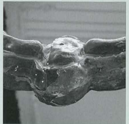
Figure d. Typical deteriorated conditions on pressed, galvanized metal pendants can include broken or missing glass (top); broken or misaligned elements (middle); and rust along the bottom of the pendant frames where water has collected (bottom). These conditions can usually be repaired.
