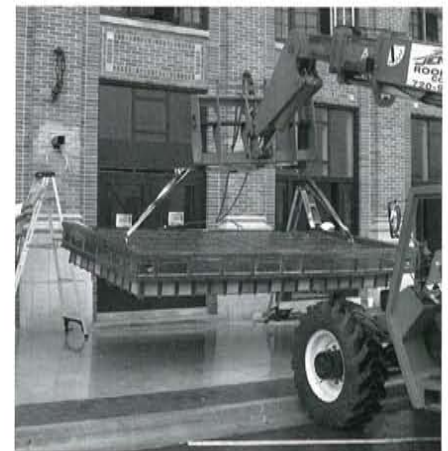
Figure 6. The installation of the new canopy required the use of a Sky Track and a special harness to ensure the protection of the copper frame. Photo courtesy of Thad Jennings, JENCO Roofing & Sheet Metal.
