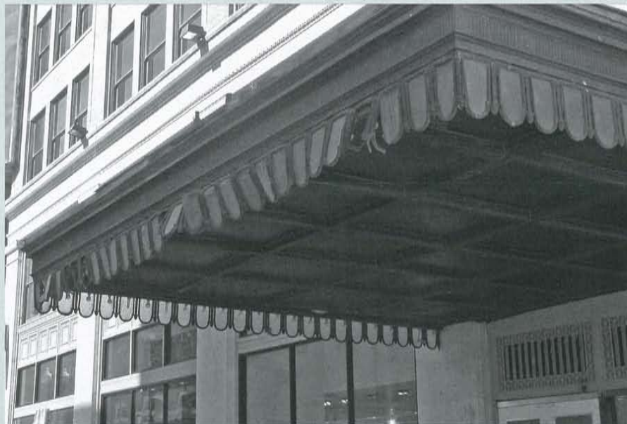
Figure a. Rust, paint failure, open joints, broken glass, or damaged and missing sections are indications that pendant frames are in need of repair.
