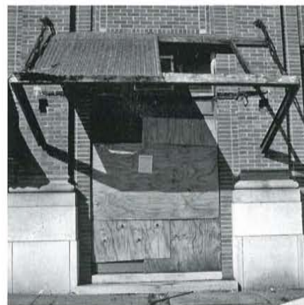
Figure 5. The east canopy entrance prior to the fabrication of its replacement. The original canopy had been replaced long ago with a simple covering that had deteriorated as well.
