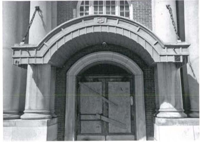
Figure 1. The Aldridge Hotel's south main entrance canopy as it existed at the start of the building's rehabilitation.
