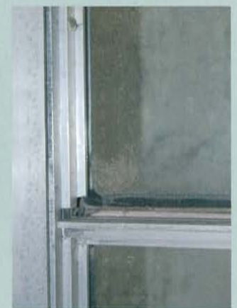
Figure b. The panes of glass were secured into the frame with aluminum glazing stops, each individually cut, drilled, and fixed in place from the inside. Here the vertical stop is in place while the horizontal is missing.
