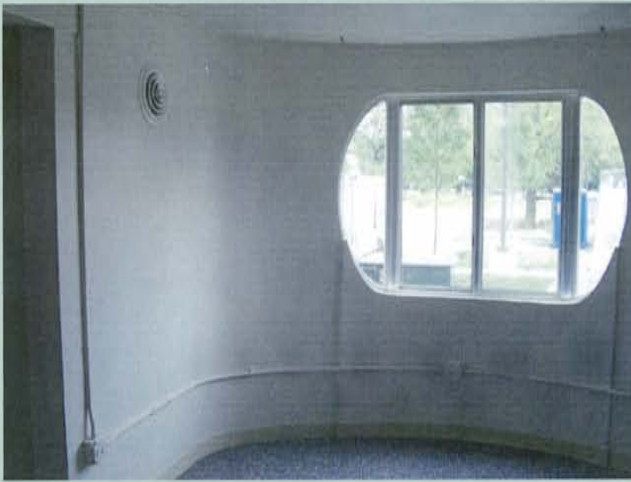
Figure e. Both interior and exterior aluminum surfaces had become dull, soiled, and oxidized as a result of traffic exhaust and air pollution. Cleaning the aluminum stabilized any further deterioration and brought back the luster of the original mill finish. (Photo: Holsten Real Estate Development Corp.)
