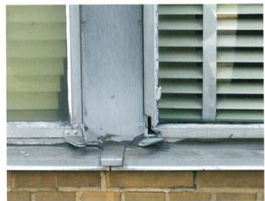
Figure 6. Deferred maintenance can result in a series of problems, such as broken hardware, cracked or missing glazing putty, and missing perimeter caulk (all shown above). All of these problems can be corrected. Note the uneven nature of the surface deposits of pollutants and grime on the mullion and sill of this window due to weathering and lack of cyclical cleaning.
