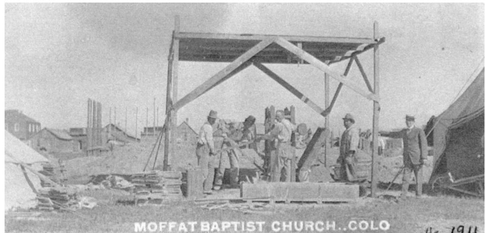
This circa 1911 photograph shows a four-man crew using a concrete block press for the Moffat church. Source: Jones, Historic Structure Assessment, 2003.
